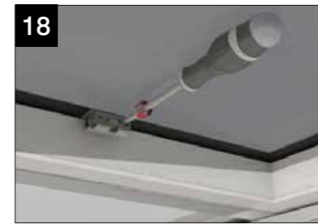
18 Using the nuts and bolts provided attach the motor bracket to the sash bracket taking care not to damage the glazed unit.
