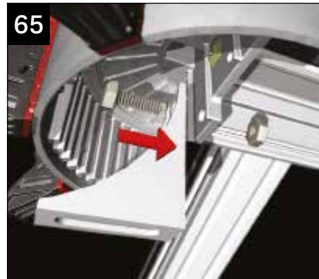
65 Fit the "L" shape PVC bracket to the underside of the radius end. Offer up the internal radius end to check the position of the bracket before tightening.
