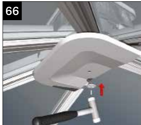
66 To fit the internal radius end capping insert the rose fixing button and tap the plastic rivet home to secure the button. On some occasions it may be preferable to test fit the ridge internal cladding prior to fitting the radius end capping.
